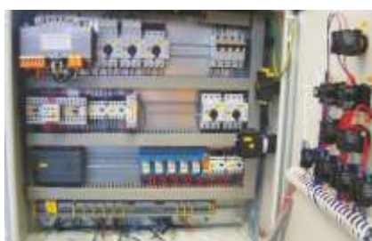
PLC controls / control cabinet
